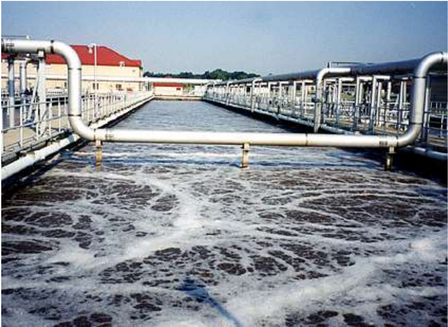
Biological Reactor with Aerated Mixed Liquor (diffused aeration)
